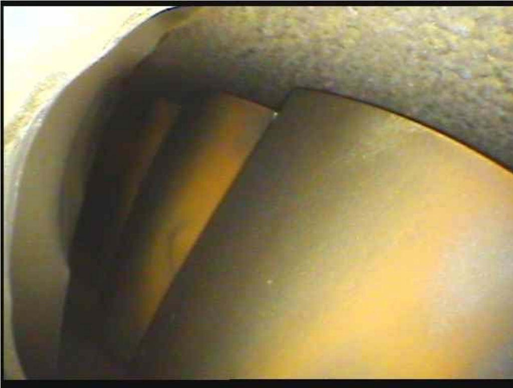
Damaged 10 stage stators.
